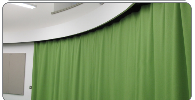
The acoustic masking drapes were hung from nine twin-2Way tracking systems designed and installed by J&C Joel.
